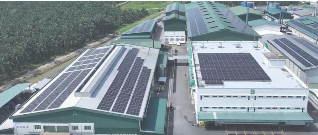
HARPS rooftop solar panels
