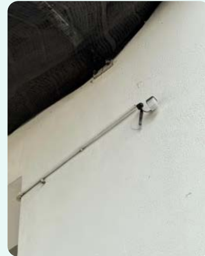
Photo sensor installed along walkway
