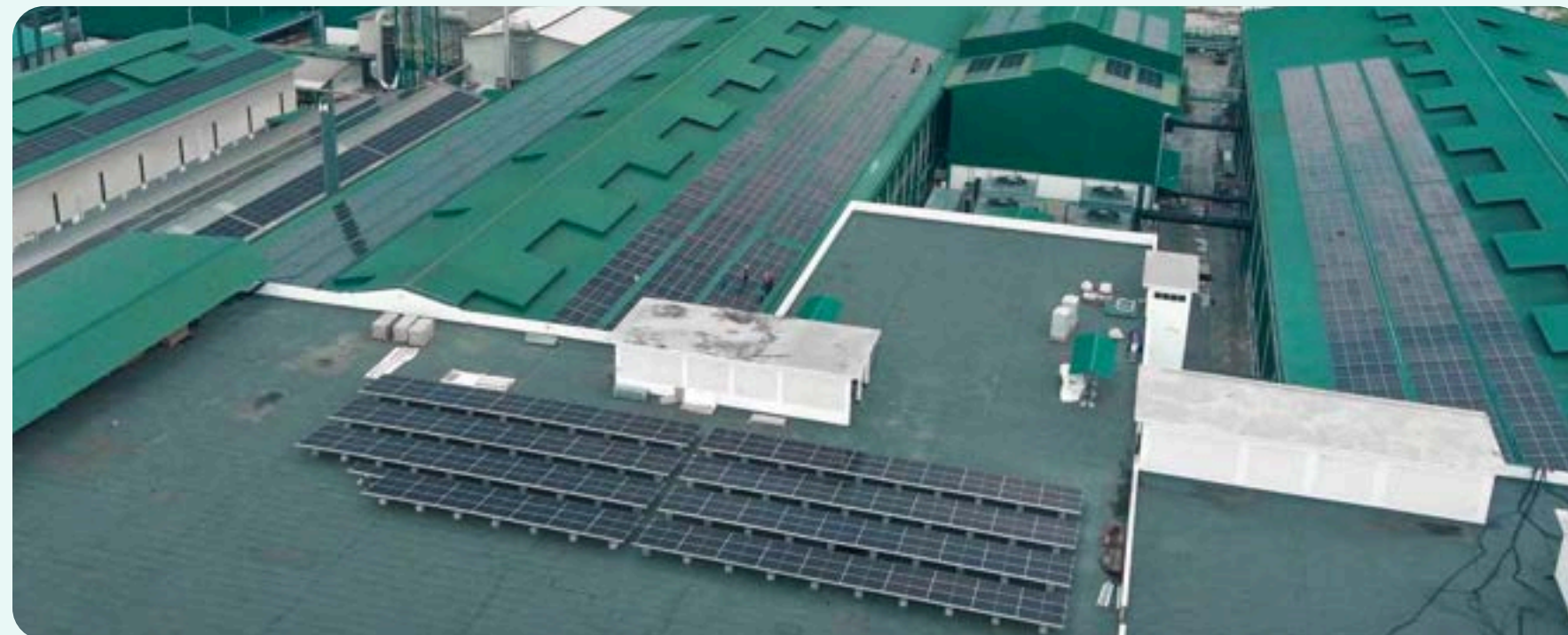
Solar panels installed on CMSB facility rooftops
